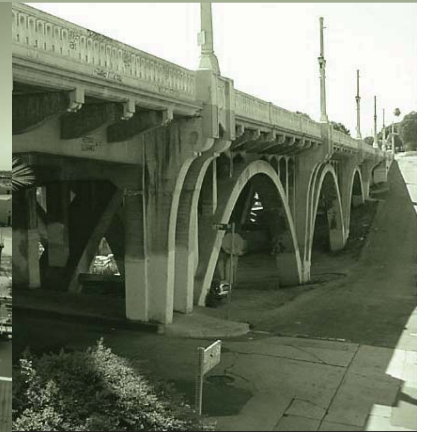
HDR worked closely with Caltrans Structures Local Assistance during the analysis and retrofit strategy phase.
